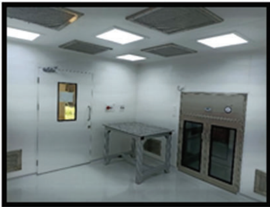
ISO-6 cleanroom with dual pass box for assembly of detectors
