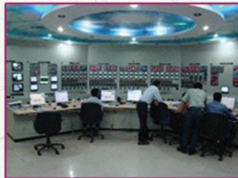
Computer-based Control & Instrumentation System for PReFRé-II
